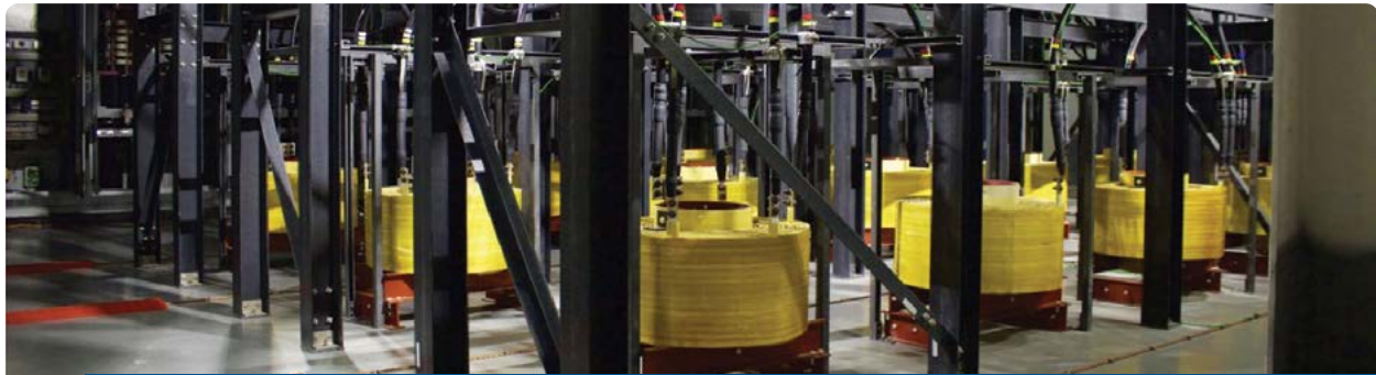
The Duke Energy Electrical Grid Research Innovation and Development center (eGRID) at Clemson can simulate the electrical grid of any country in the world to test how cities would manage cyberattacks to power infrastructure
